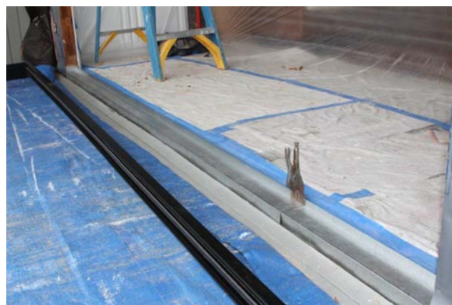
Metal pan flashing installation at subfloor prior to new sliding glass door replacement
