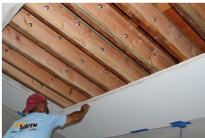
Interior joist repair/replacement at cantilevered balcony reconstruction - city building permits required for this project
