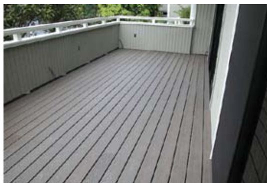
Balcony with a gapped decking finished floor
