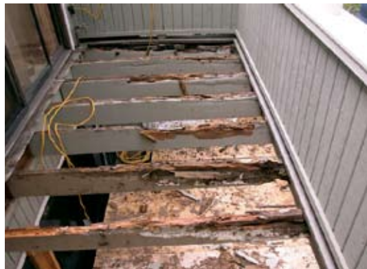
Severe decay in cantilevered floor joists
