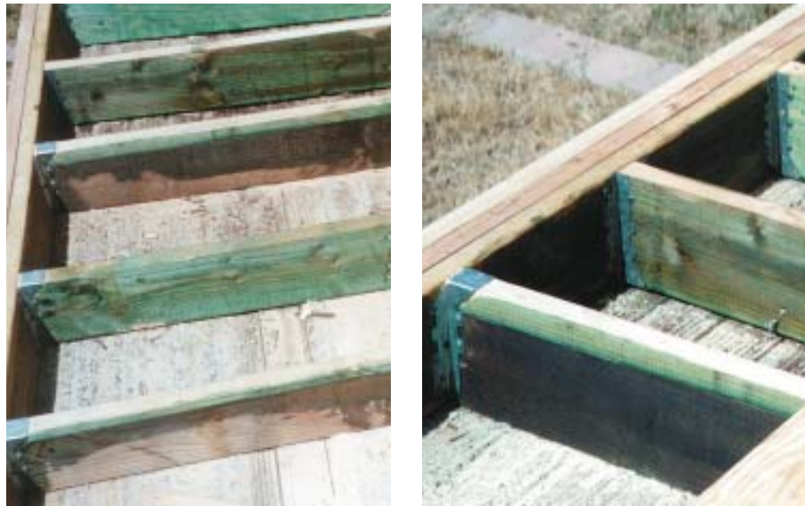
Figure 4. Joists that are too far gone to repair must be replaced between the wall plate and the new double rim joist (left). The rim hangs at the ends of the intact cantilevered joists on upside-down joist hangers. The replaced “cripple joists” are hung conventionally (right).
