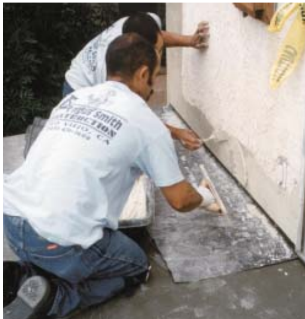
Figure 7. Stucco siding repairs follow the original three-layer process of scratch coat, brown coat, and color coat. A narrow strip of the sheet-metal flashing is left exposed to allow crack-free movement between wall and deck.
