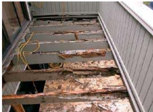
Severe decay in cantilevered floor joists
